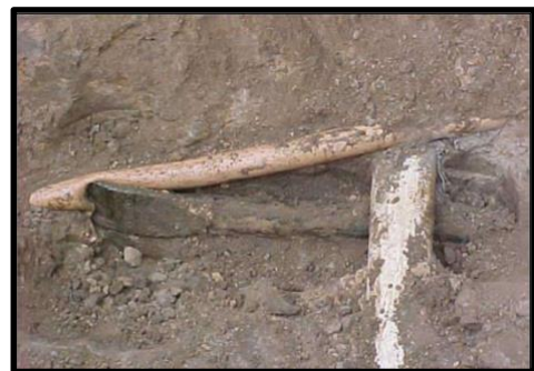
Figure 4: Class 2 Cross Bore. Communications HDD intersects sewer lateral then gas line
