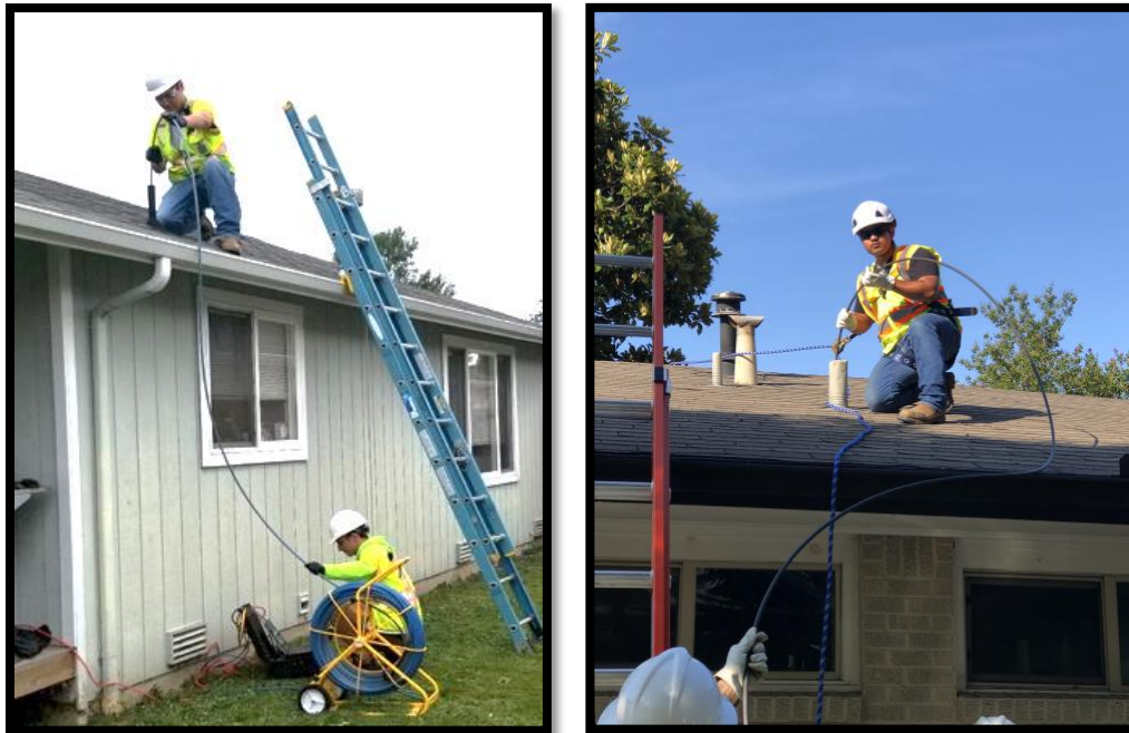
Figure 20: Roof vent inspection with manual push camera. Fall protection must be used according to safety regulations.
