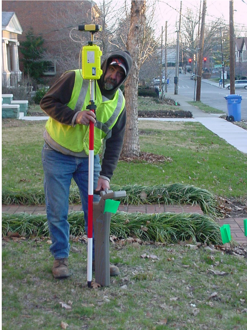
Figure 11: CCTV Field inspector captures lateral line trace with sonde receiver and Wireless GPS Mapping Stick
